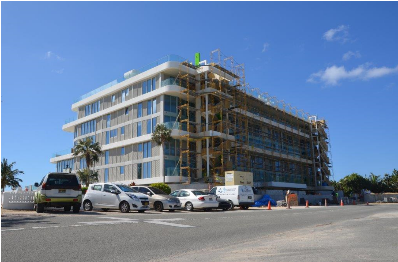
The Tides development in South Sound is one of the large projects under construction in Grand Cayman.
