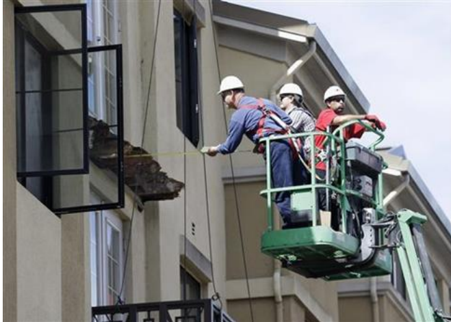
Workers inspect damage from a fallen balcony that resulted in the deaths of eight Irish tourists. Negligence in this case can apply to virtually everyone involved with the building, the San Francisco Examiner determined. Credit SF Examiner.
