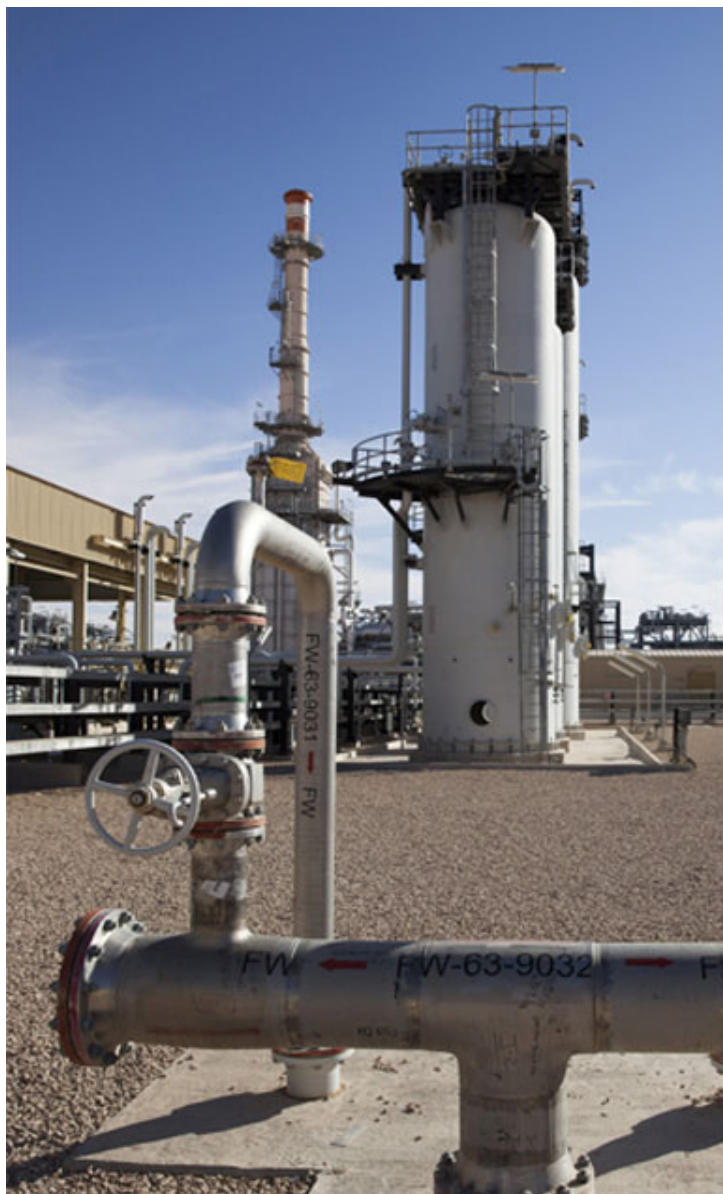
El Merk Facility, Algeria
