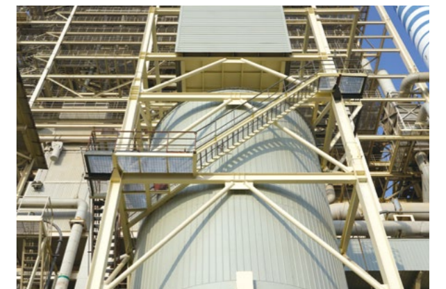
At Ma'anshan Dangtu Power Generation Co., Ltd., a 168-hour trial operation has been completed as scheduled for the No. 2 drying tower system of the zero-wastewater discharge transformation project.
