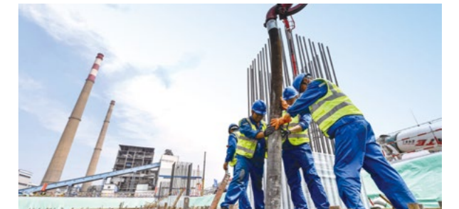
Construction of the two 660MW heating units at Hebei Douhe Thermal Power Plant
