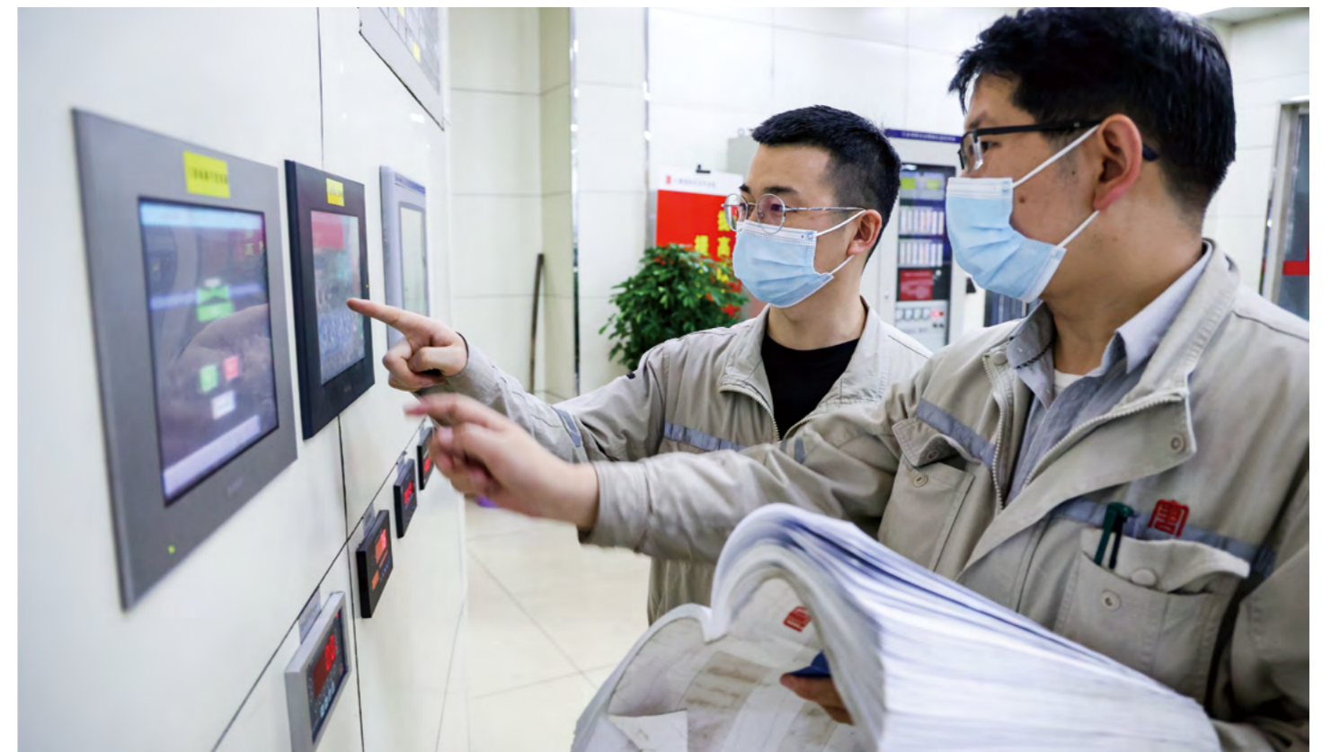
Ensuring high-quality power supply through meticulous control of indicators
