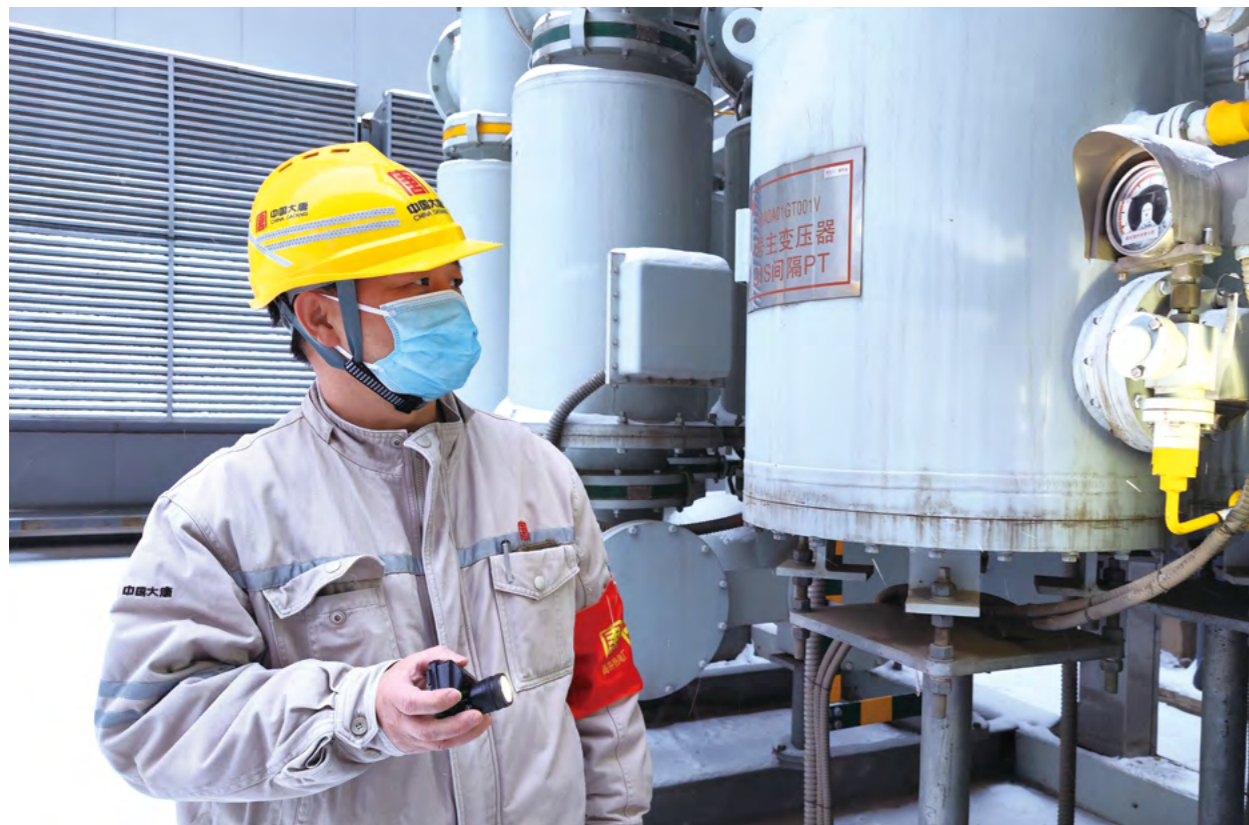
An inspector from Gaojing Thermal Power Plant conducts an outdoor equipment inspection
