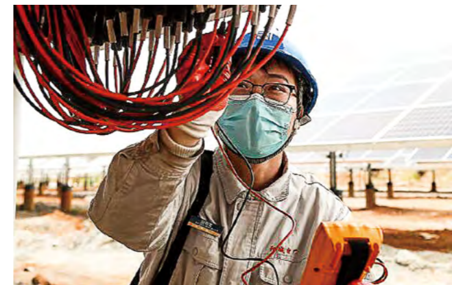
Shanxi Branch carries out maintenance of the photovoltaic power station to ensure its safe, stable and efficient operation.
