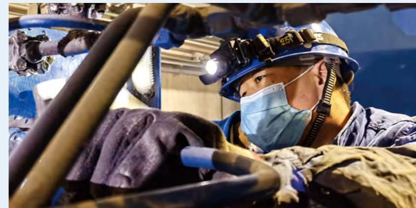
Hebei Zhangjiakou Power Plant inspects equipment safety to ensure power supply for Beijing 2022.
