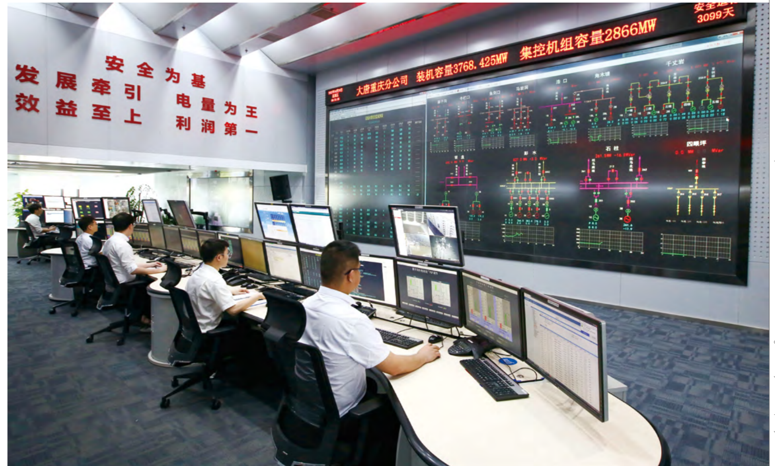
The multi-energy centralized control center at Chongqing Branch
