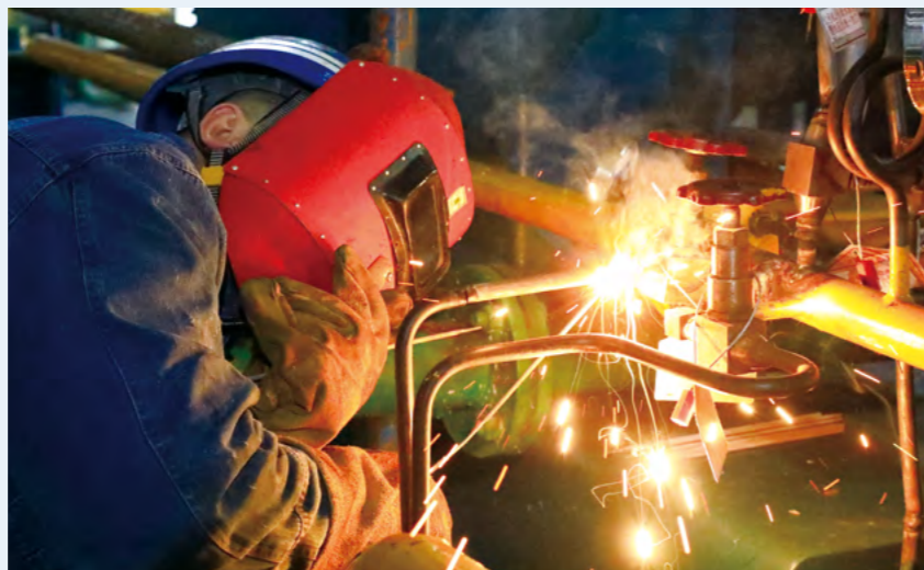
Hebei Baoding Thermal Power Plant conducts generating unit inspection and maintenance to comprehensively investigate potential equipment hazards.
