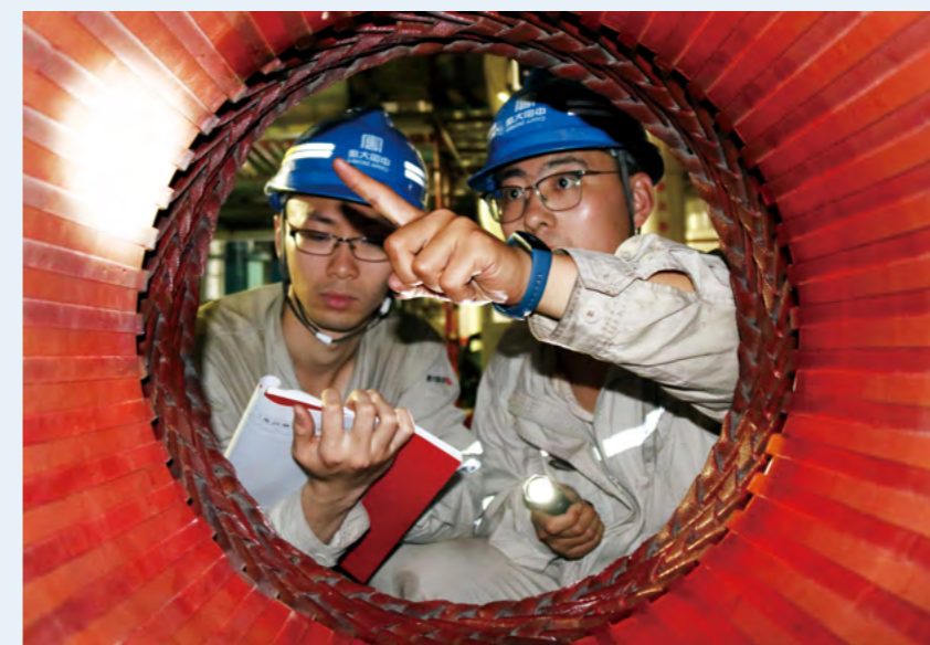
Tianjin Panshan Power Generation Company conducts equipment inspection and maintenance.
