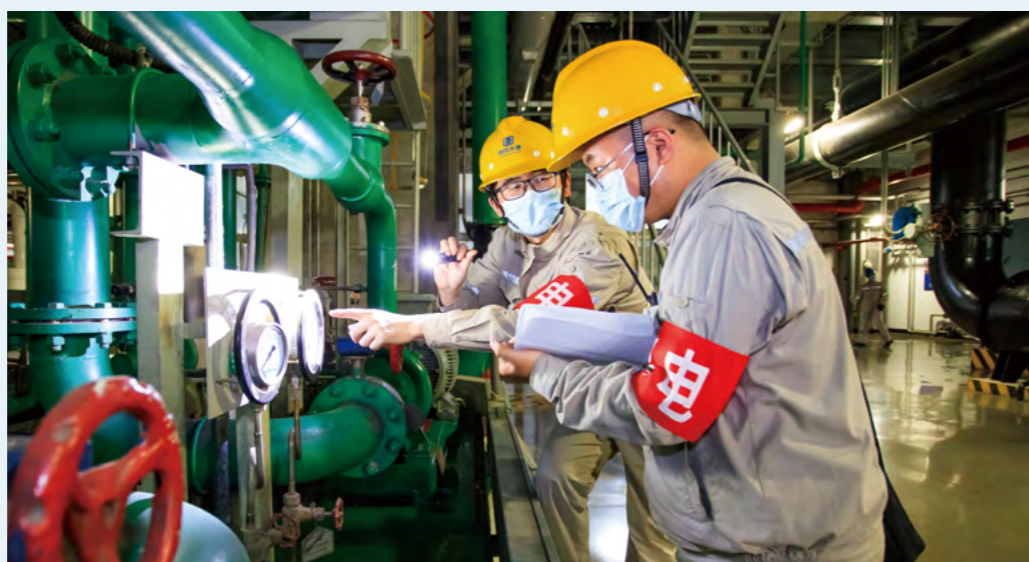
Inner Mongolia Tuoketuo Power Generation Company strengthens equipment inspections.
