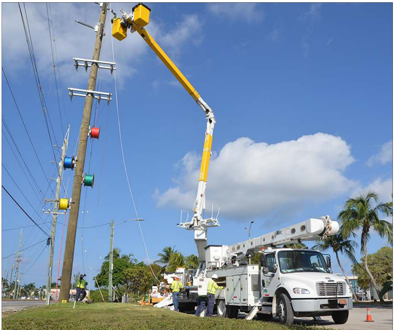
A number of major upgrades to the Company’s transmission and distribution system were carried out in 2021 to accommodate new residential and commercial customers.
