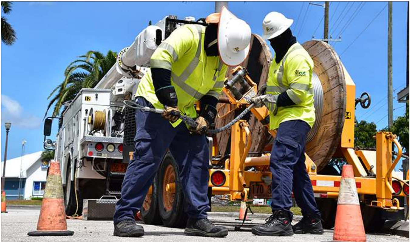
The Company's employees are provided with the highest rating of safety clothing and equipment to combat the extremely warm and humid conditions in the Cayman Islands.
