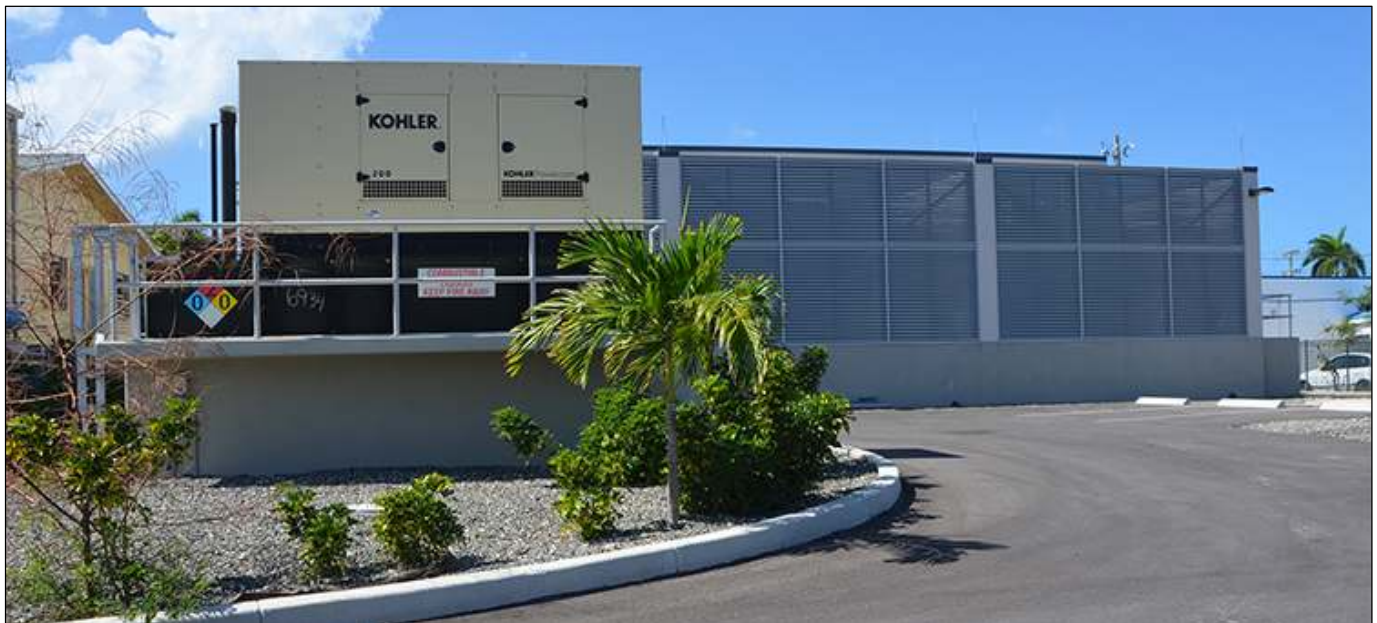
The Seven Mile Beach Substation on West Bay Road is expected to be commissioned in 2021.
