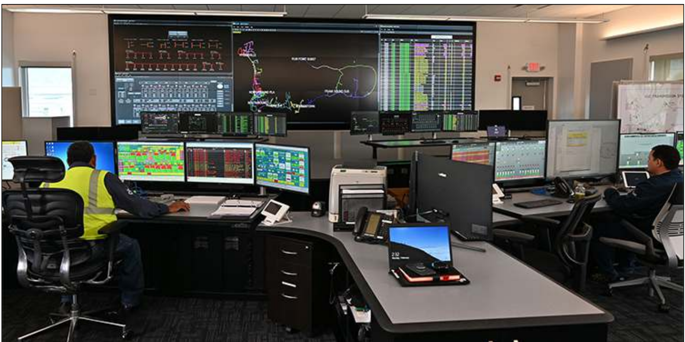
The Company's upgraded Control Room in the newly constructed Technology Centre.
