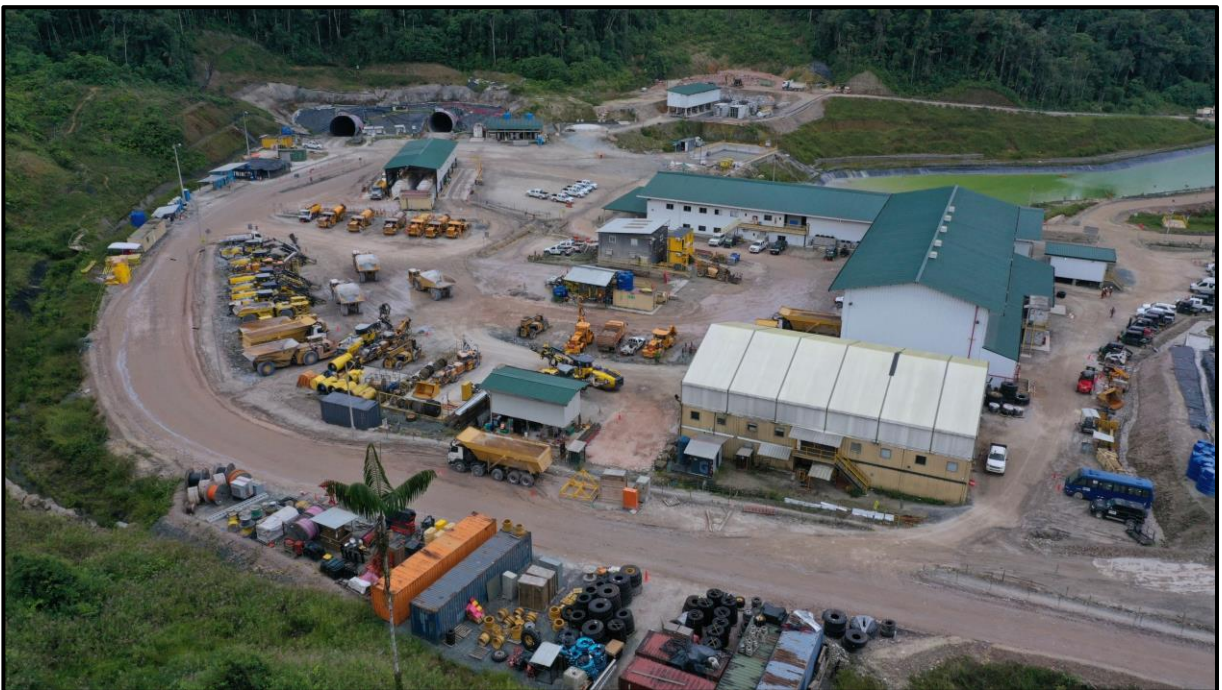
Figure 2. Portal platform as at September 2019
