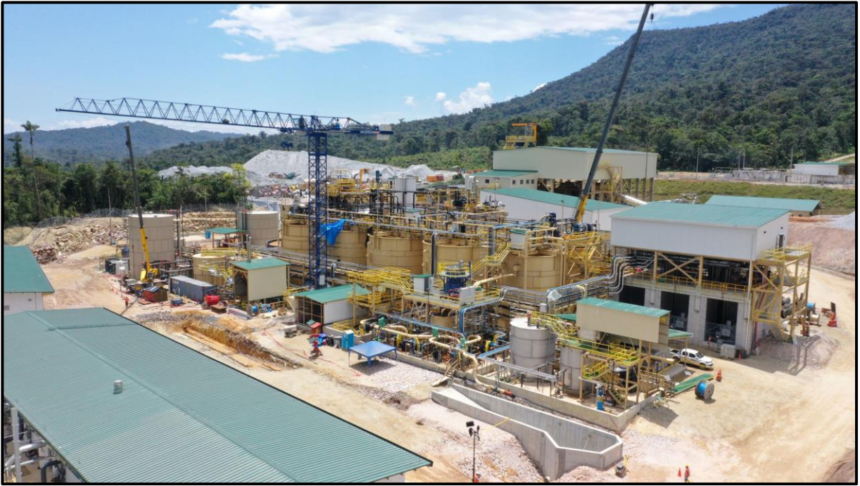
Figure 3. Process plant as at September 2019
